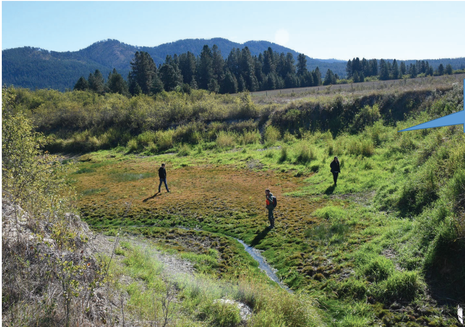
Photograph 8. View of the sediment plume and failing/sluffing slopes on the downstream face of the Maslonka Dam in Perkins Slough. This is the downstream face of the dam and field crew are standing well below the OHWM on September 16, 2021. View is generally southeast and downstream. Note extensive cattle tracks in the Slough channel bottom.
