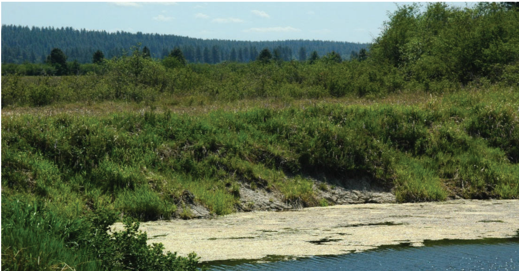
Photograph 11. Channel Bank Scour and Slope Failures At and Below the OHWM on the Upstream Face and Immediately Upstream from the Maslonka Dam On September 16, 2021. View is southeast and upstream.
