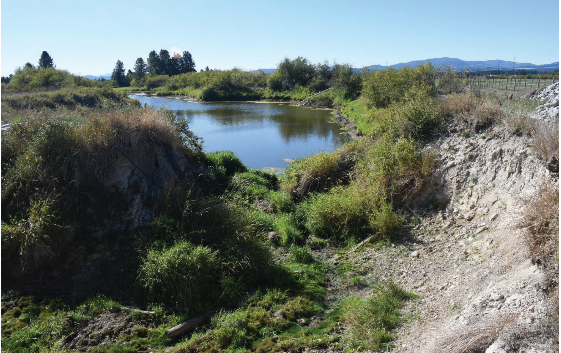
Photograph 6. Close-Up of the Breach in the Maslonka Dam on September 21, 2021. View is southwest and upstream. Note the channel bank instability (scour erosion) on the right side (Slough left looking downstream) of the Photograph.
