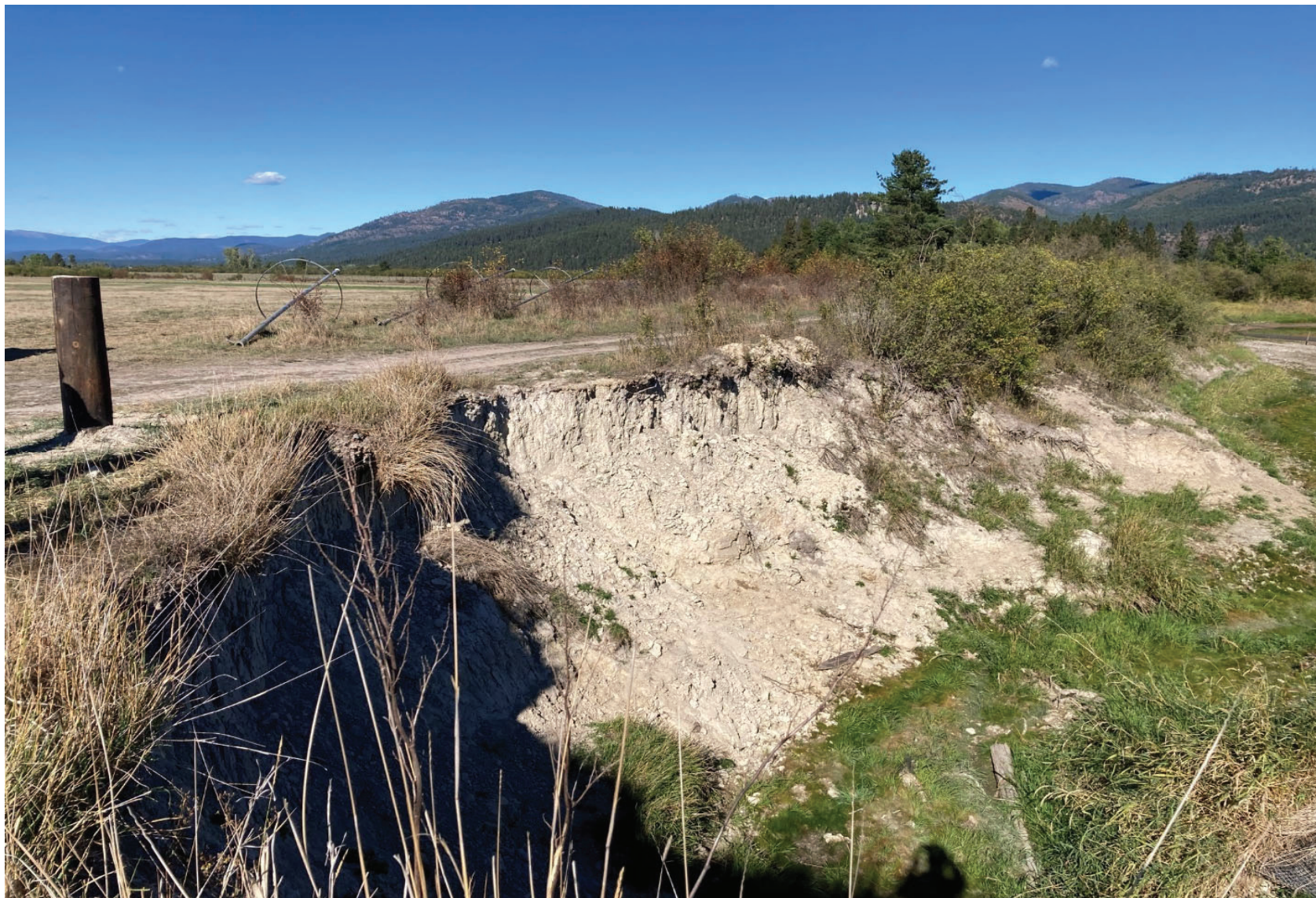
Photograph 10. Close-Up of Scour Slope Failures on the North (Slough Left) Side of Perkins Slough, Downstream of the Maslonka Dam on September 16, 2021.
