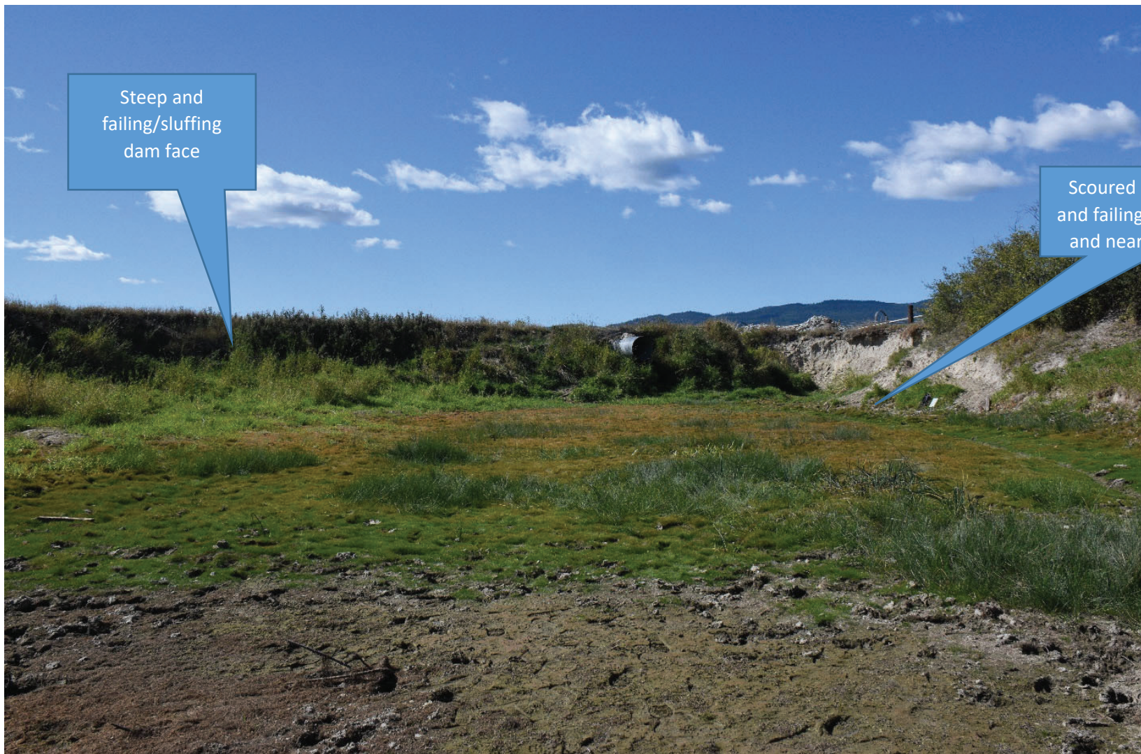
Photograph 9. Scour and Sluffing Areas On and Near the Downstream Face of the Maslonka Dam. View is west and upstream.
