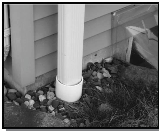
Sources of stormwater in the collection system may include building downspouts connected directly to the system (photo: MMSD).
