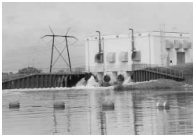
Source: The S-9 structure that back-pumps contaminated water from the C-11 canal in Broward County into the Everglades. Photo by author, September 2003.
