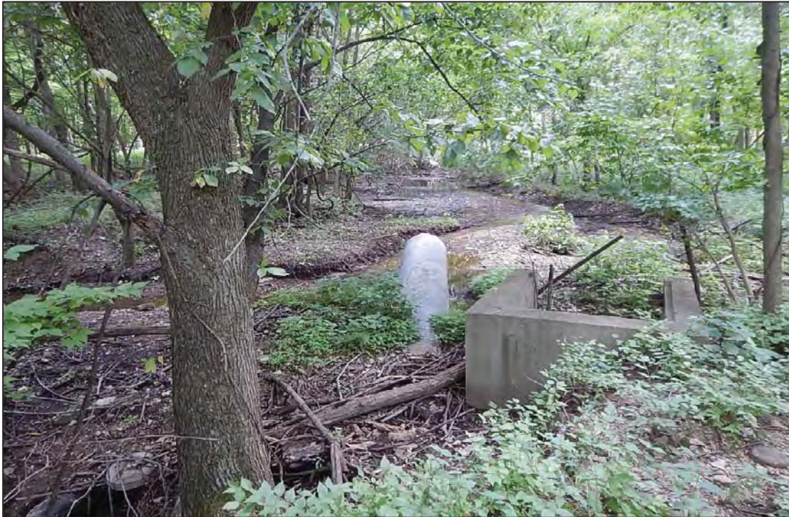
PHOTO 3: View to west of structures in place at eastern end of drainage ditch.
